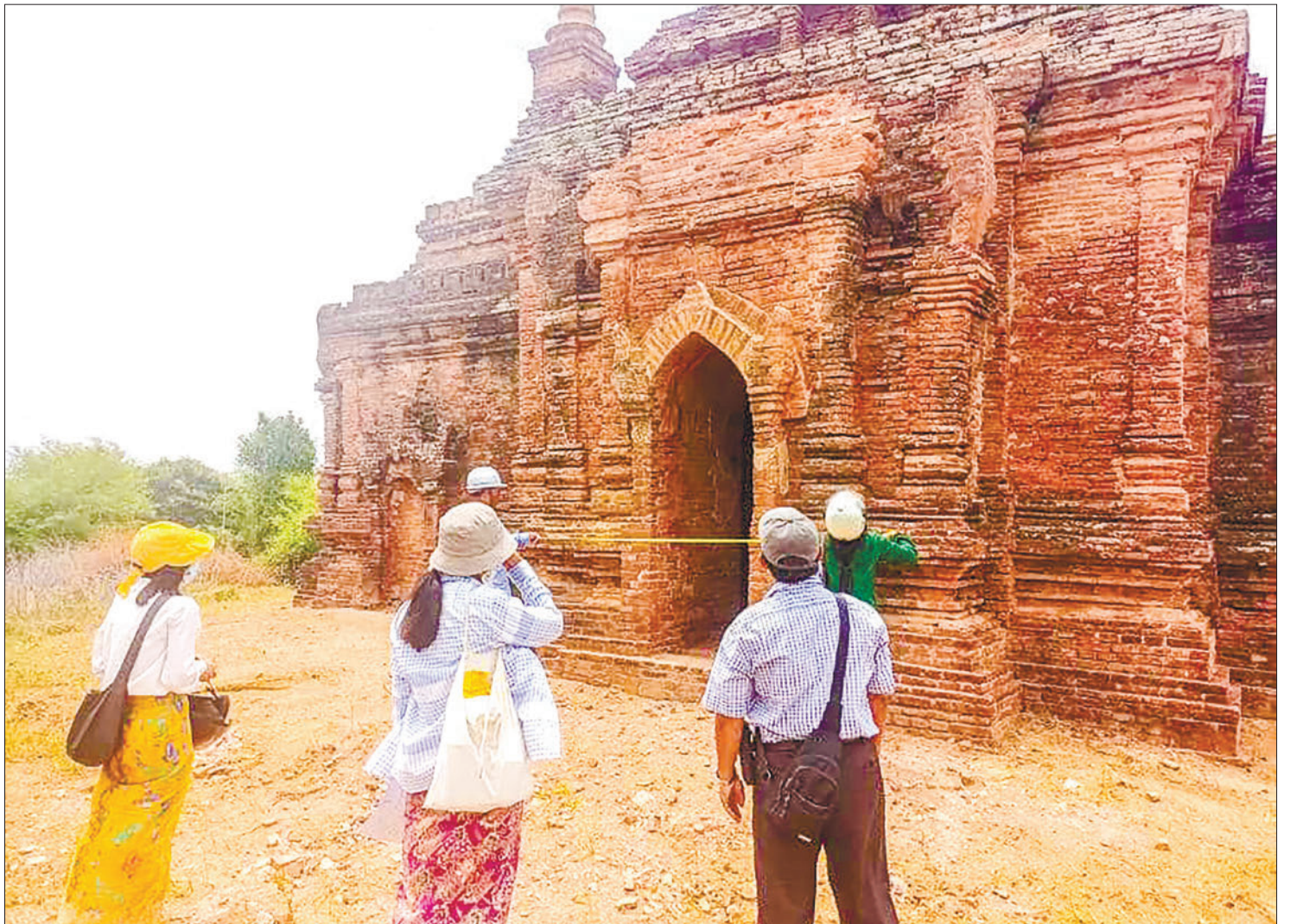
Restoration efforts for Cyclone-damaged ancient buildings and pagodas in Bagan Archaeological Zone in progress.
