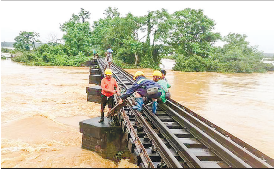
Engineers from Myanmar Railways conduct assessments to evaluate potential structural damage to the bridge on the Bago-Mawlamyine railways line.
