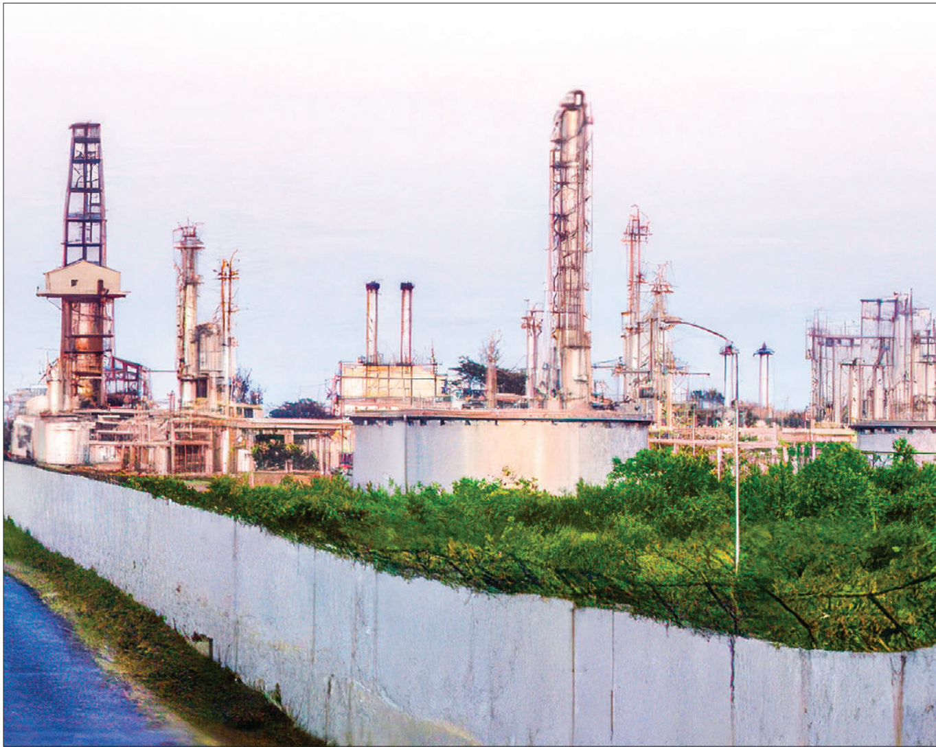
The photo shows Thanbayakan Oil Refinery run by the Myanma Petrochemical Enterprise.
