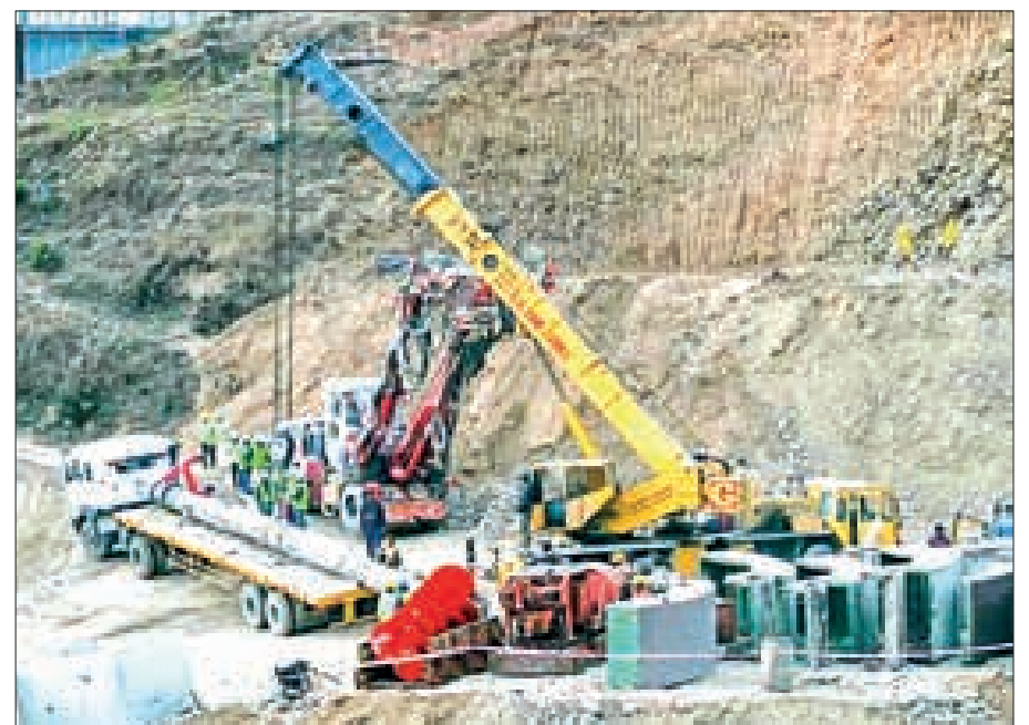
Rescue personnel work at the mouth of the collapsed under construction Silkyara tunnel in the Uttarkashi district of India's Uttarakhand state, on 25 November 2023. PHOTO: AFP
