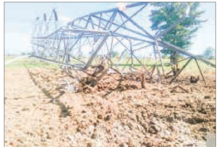
230 KV Thayagon-Kamanet-Baider electricity transmission tower destroyed by terrorists.
