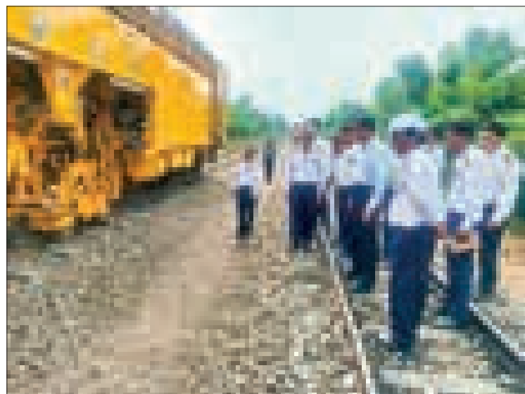
Deputy Minister for Transport and Communications U Aung Myaing inspects the ongoing upgrade of the Toungoo-Nay Pyi Taw railway section on 1 December 2023.
