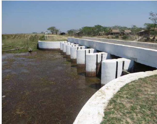
Sluice gate for irrigation water
