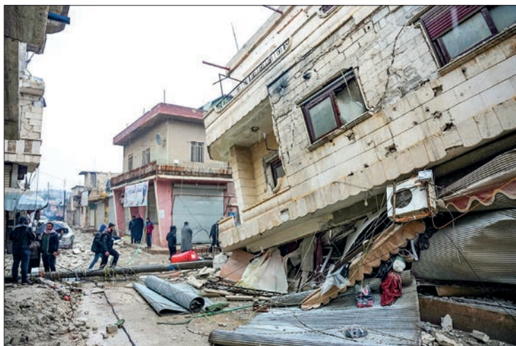
Residents walk along a collapsed building following an earthquake in the town of Jandaris, in the countryside of Syria's northwestern city of Afrin in the rebel-held part of Aleppo province, on 6 February 2023. PHOTO: AFP
