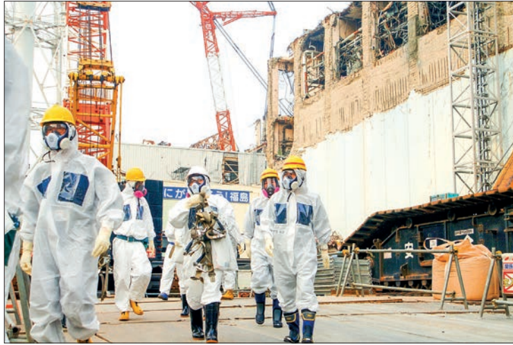
In this 17 April 2013 file photo, IAEA experts depart Unit 4 of TEPCO Fukushima Daiichi Nuclear Power Station as part of a mission to review Japan's plans to decommission the facility. PHOTO: REPRESENTATIVE IMAGE/ IAEA
