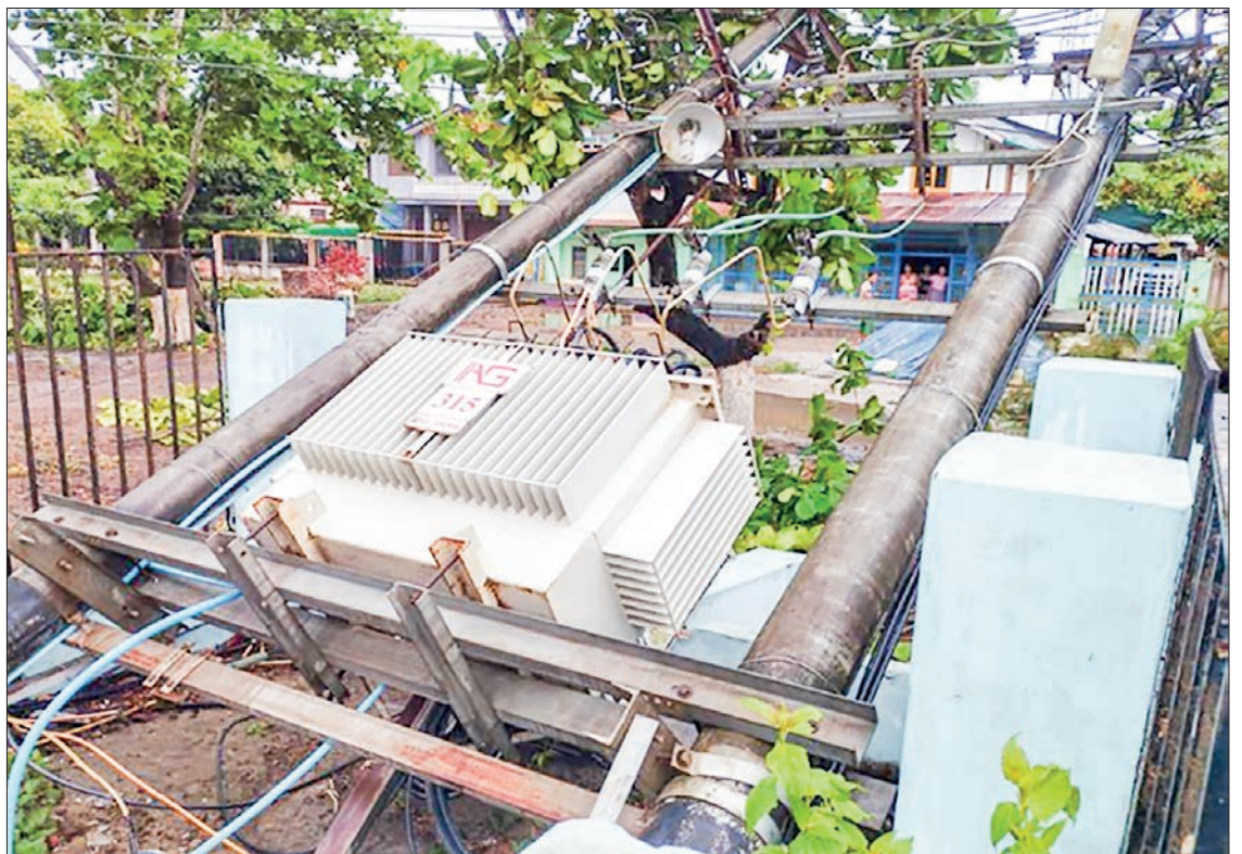
A transformer fell in residential ward in Gwa Township of Rakhine State on 14 May.
