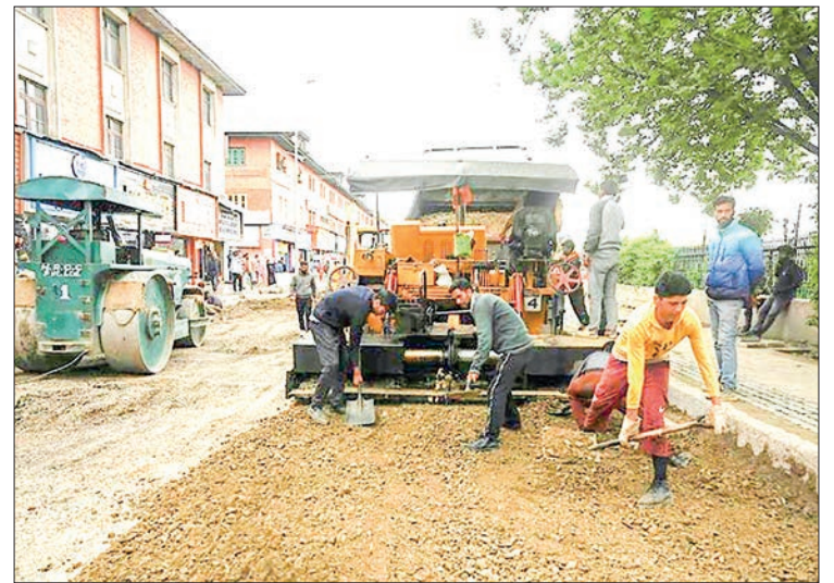
Labourers work on a road along a street under the Smart City project ahead of the G-20 meetings, in Srinagar on 26 April 2023. PHOTO: AFP
