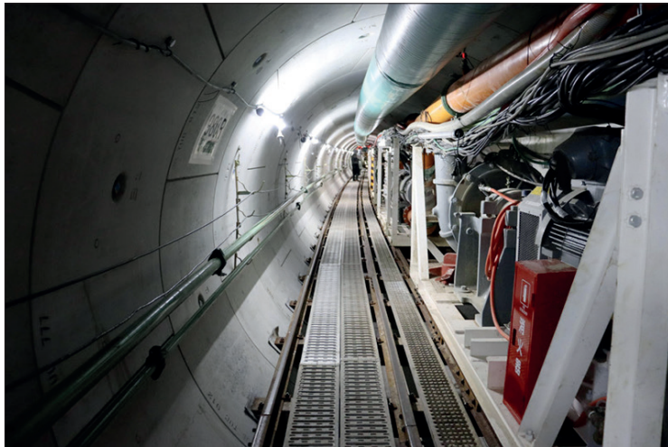
Photo shows an undersea tunnel to be used to discharge treated water from the crippled Fukushima Daiichi nuclear power station in Japan's northeast. PHOTO: TOKYO ELECTRIC POWER COMPANY HOLDINGS INC./KYODO
