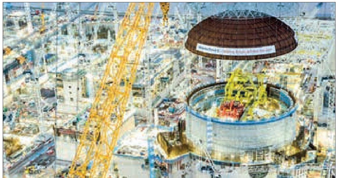
An EDF handout showing the steel dome being installed over Hinkley Point C's reactor 1. PHOTO: HANDOUT/AFP
