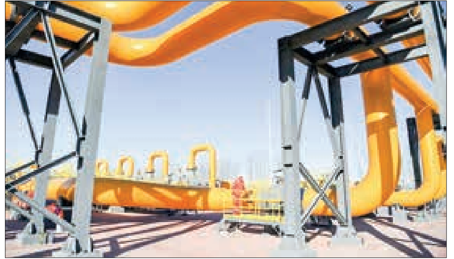
A staff member works at the Yongqing compressor station of the Changling-Yongqing section of the China-Russia east-route natural gas pipeline in Yongqing County, north China's Hebei Province, 3 December 2020. PHOTO: XINHUA
