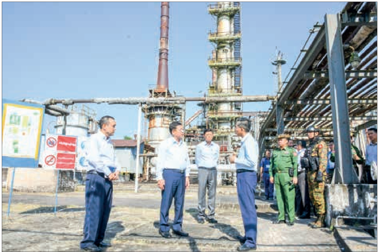
SAC Chairman Prime Minister Senior General Min Aung Hlaing inspects No 1 Oil Refinery (Thanlyin) in Yangon yesterday.
