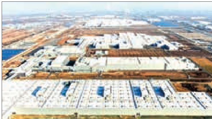
Aerial photo taken on 28 December 2021 shows the new Tiexi Plant of BMW Brilliance Automotive (BBA) under construction in Shenyang, northeast China's Liaoning Province. PHOTO: YANG QING/XINHUA
