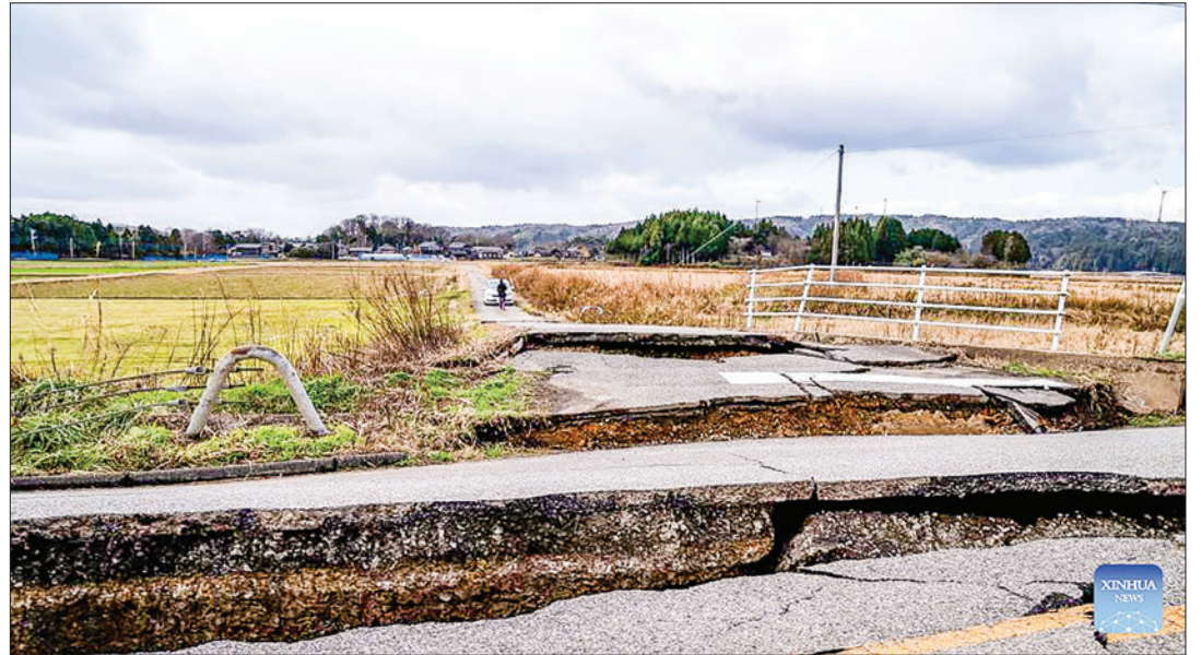
This photo taken on 2 January 2024 shows a road damaged by earthquakes in Hakui, Ishikawa prefecture, Japan. PHOTO: XINHUA
