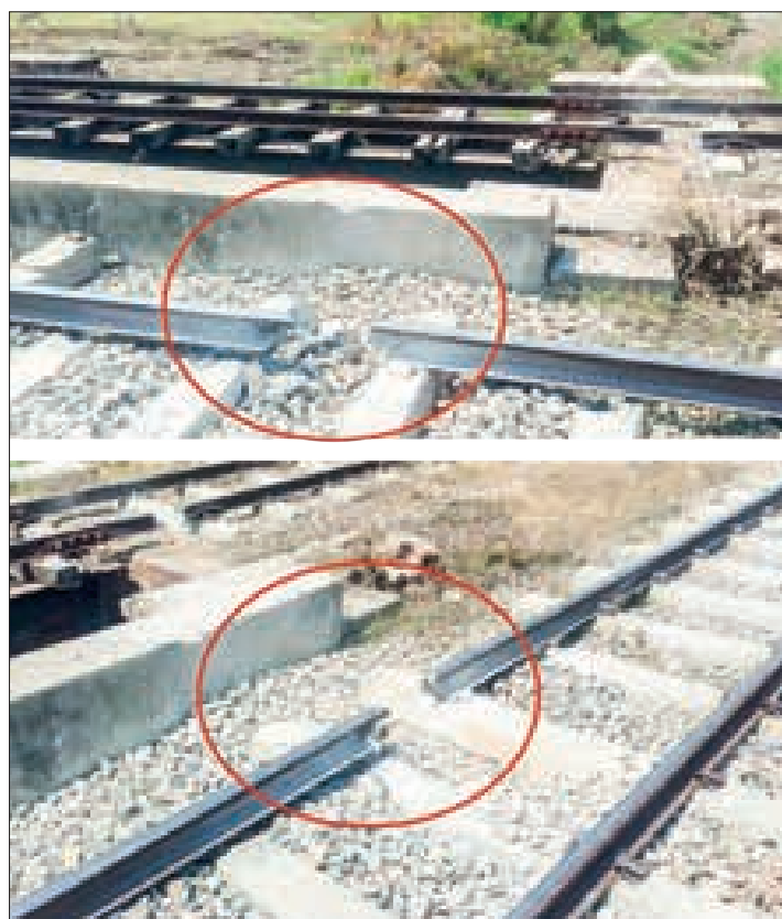
The explosion places of railway lines between mileposts 353/24 and 354/1 on the Yangon-Mandalay railways destroyed by terrorists.
