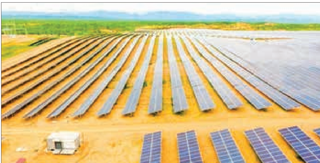
The photo shows the generation of electricity from solar power.
