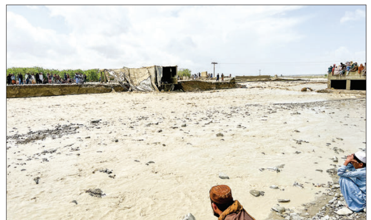
Residents gather beside a collapsed bridge due to flood waters following heavy rains in Pishin district on 15 April 2024. PHOTO: AFP
