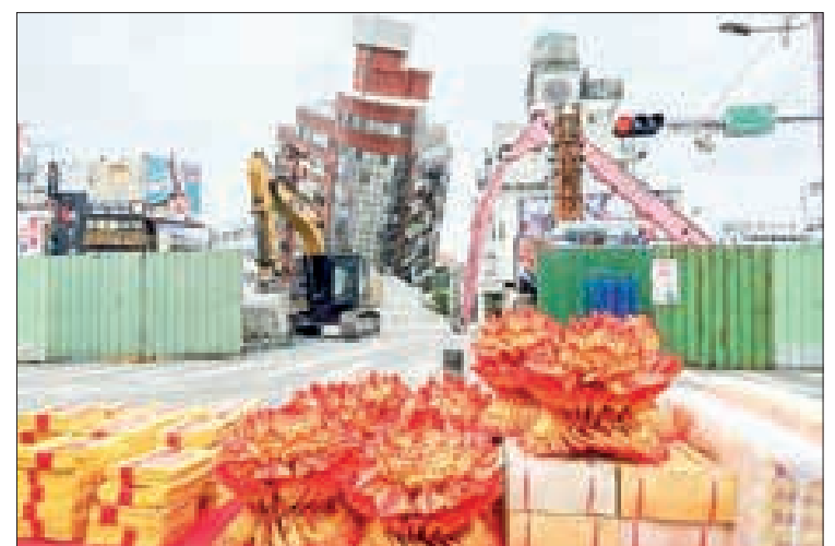
Paper money is placed on a table as an offering before demolition work begins on a precariously tilting building in Chinese Taipei's Hualien. PHOTO: CNA/AFP
